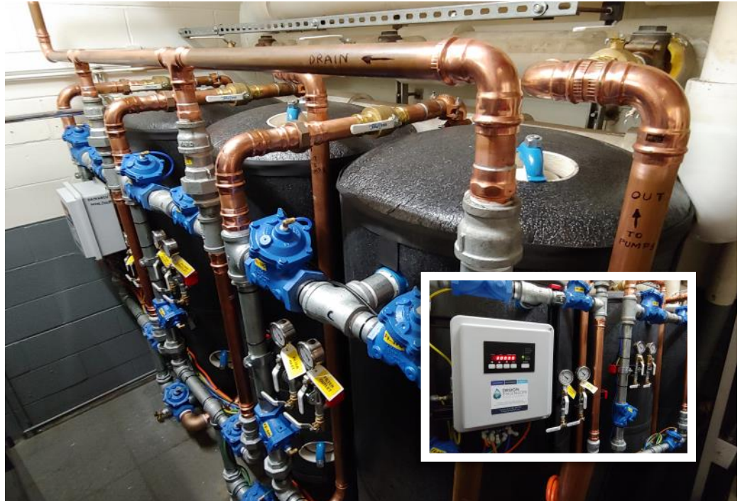
This is the new computer controlled water filtration system that serves the domestic hot and cold water supply. The water quality is monitored continuously and the system flushes automatically on a weekly basis.
