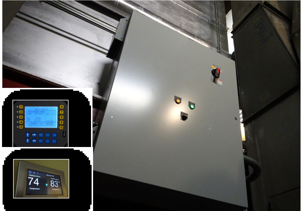
One of two new computerized control panels that operate the cooling towers. The inset above left is the control panel for the continuous water quality sensor, below that is the readout of the cooling tower status that is installed in the concierge station.
