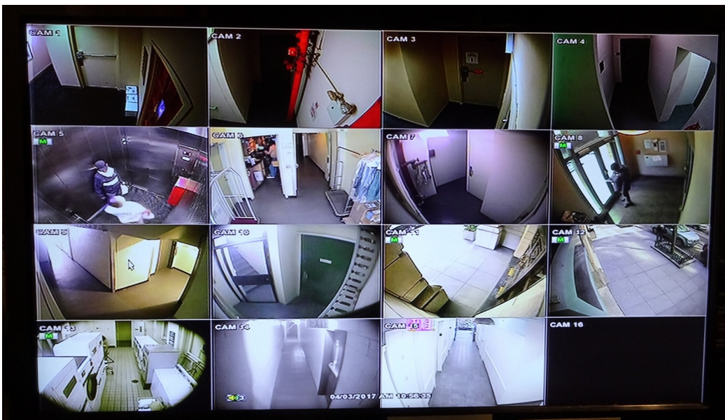
The concierge station security camera monitor displays all coverage areas. Movement or sound in some areas will trigger an alarm.
