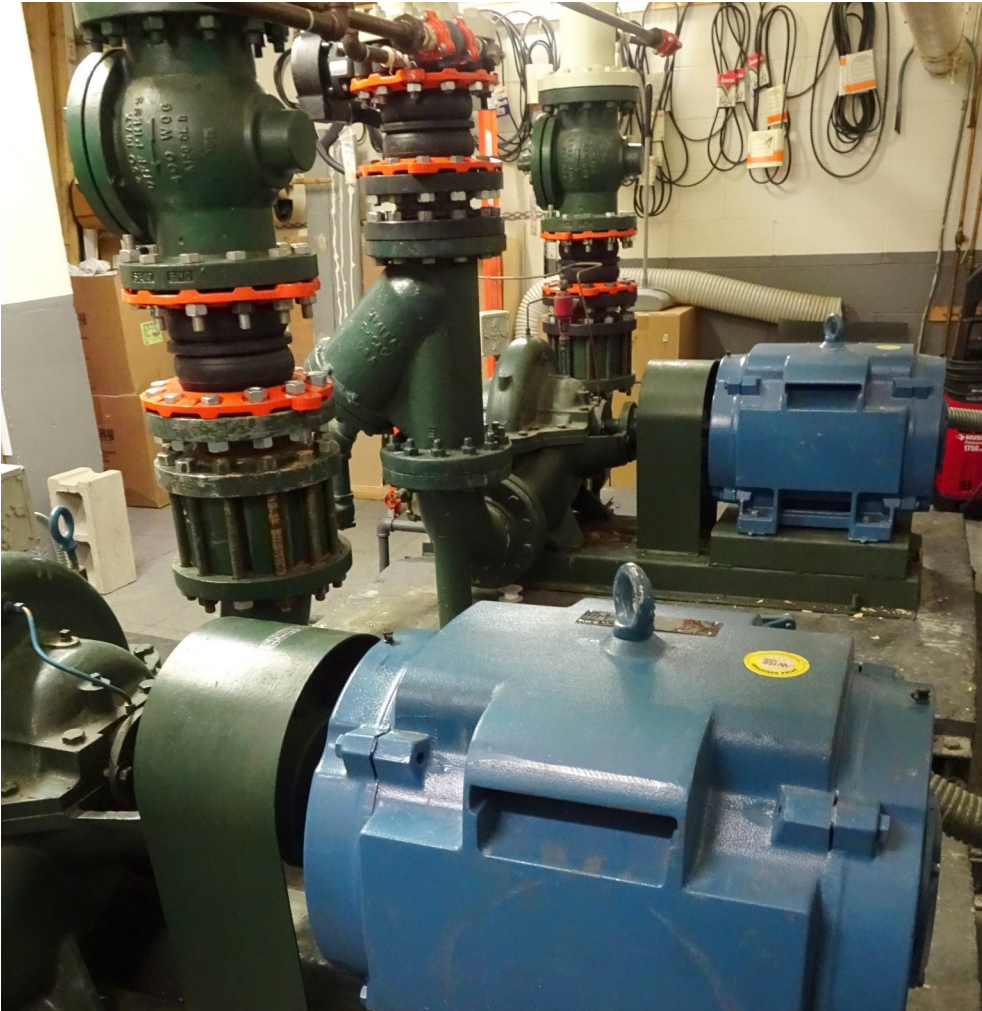
New variable speed, computer controlled motors are energy efficient and can instantly cover for failure in the other unit.
