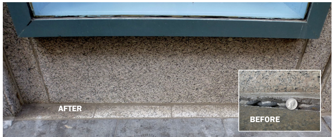
Shifting of some of the granite façade stones was not structurally significant but caused water penetration and visible cracks in a few places at the first floor level. It is possible that a small earthquake or work on the Second Avenue Subway line could have caused this problem.
