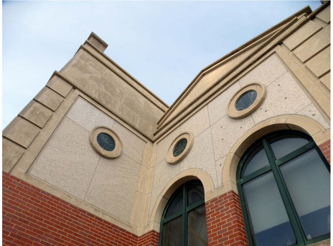
Coping consists of the capping or covering of a wall. The façade work done over the last few years did not discover problems with the stones on the setback wall tops and granite facing at the top of the building. Many new pins were inserted to provide maximum security of the coping.
