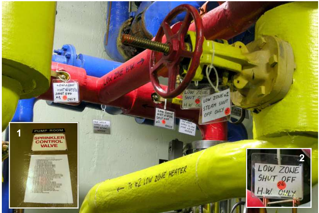
The newly tagged, numbered and painted valves and pipes make it much easier to locate a specific valve. The door to each equipment room has a list of valves (inset #1) and each valve has a description and number (inset #2).
