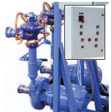
Our system will have three pumps instead of the two shown in the illustration. The computerized control panel is shown in the inset.
