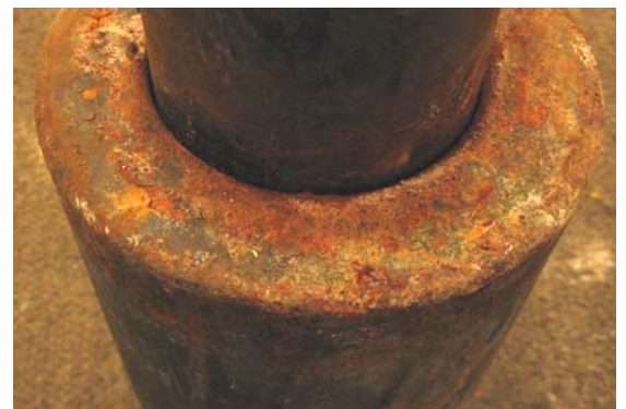
This is the actual expansion joint described in the story at left. These joints are essential in long pipe strings. They have internal rings designed to keep water from escaping. However, it is a mechanical device and like any other, has the potential for failure.
