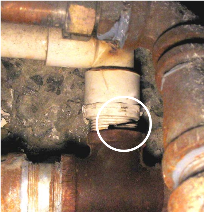
The plastic HVAC drain pipe was connected to a metal pipe. For some reason, the plastic pipe cracked and broke causing a leak whenever the unit created condensate. This crack could not be repaired since the unit owner would not allow access. The leak was stopped temporarily by shutting the unit down. It is now being repaired.
