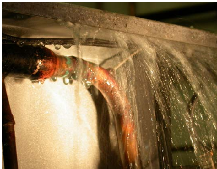
The failure a copper solder joint in an HVAC unit illustrates the fact that water damage is often the result of accidental failure of otherwise well-maintained systems. This unit is one of many hundreds in the building and the only one ever to have this kind of failure. There is no one to blame for one random failure and the cost of replacing all HVAC units because of this one failure would be unacceptable. This is why you need homeowner's insurance.
