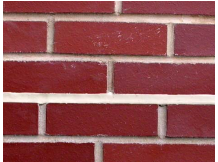
Above the Atrium, on the West wall at the third floor level, a sample of what the façade remediation would actually look like has been installed. Two different possible techniques have been proposed. The costs and benefits of each are being carefully considered.
