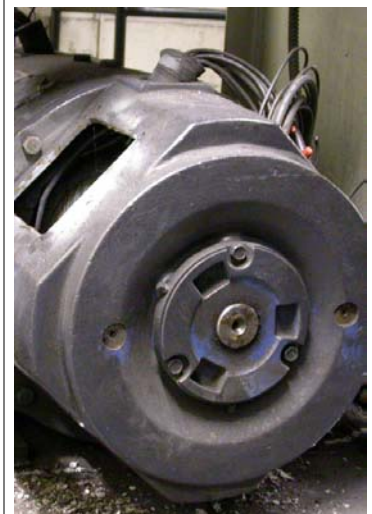
The generator burned out and must be replaced.
