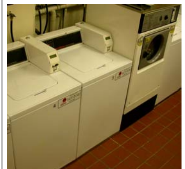
Our current laundry room will be completely renovated, new machines, new floor, new ceiling.
