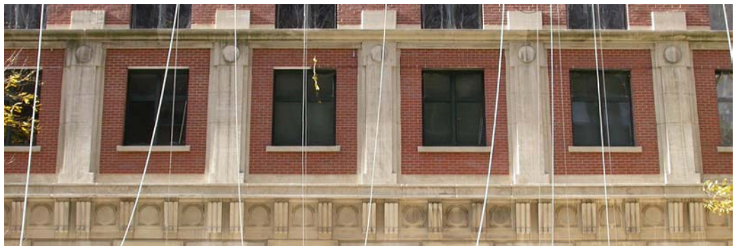
The photograph of the third floor shows the finished product of the façade renovation. Work is progressing as planned.
