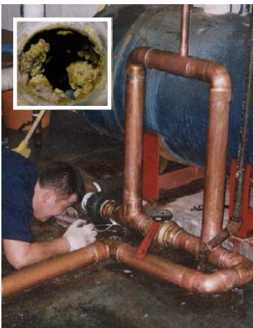
Victor, our very capable new handyman soldering new copper pipes. Inset shows the corrosion that almost completely blocked some of the pipes and valves.
