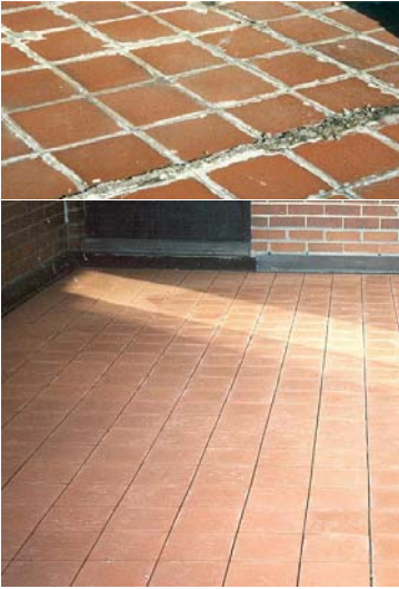
The badly damaged and leaking terraces were stripped to the foundation and completely rebuilt.
