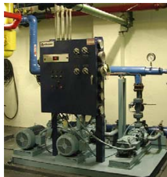
Main water pumps
