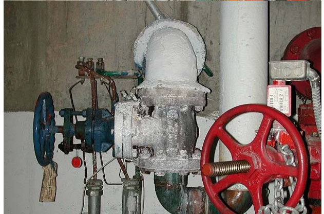
Main water shut-off valve. Top photo the serious state of corrosion. Above, the valve has been insulated and fully checked and cleaned. All valves in this room were serviced.
