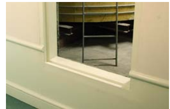
The 5,000 gallon tank for fire emergency has a proper door frame designed to contain a flood of water should a system cause a major flood.
