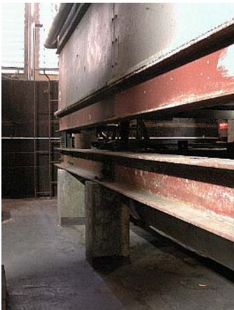
The cooling tower contains thousands of gallons of water. The floor was never waterproofed. This must be done to protect against flooding of units below.
