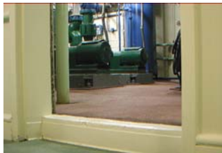
HVAC room does not have a flood stopping door frame. A failure of a major system could cause water to flood hallways and units below.
